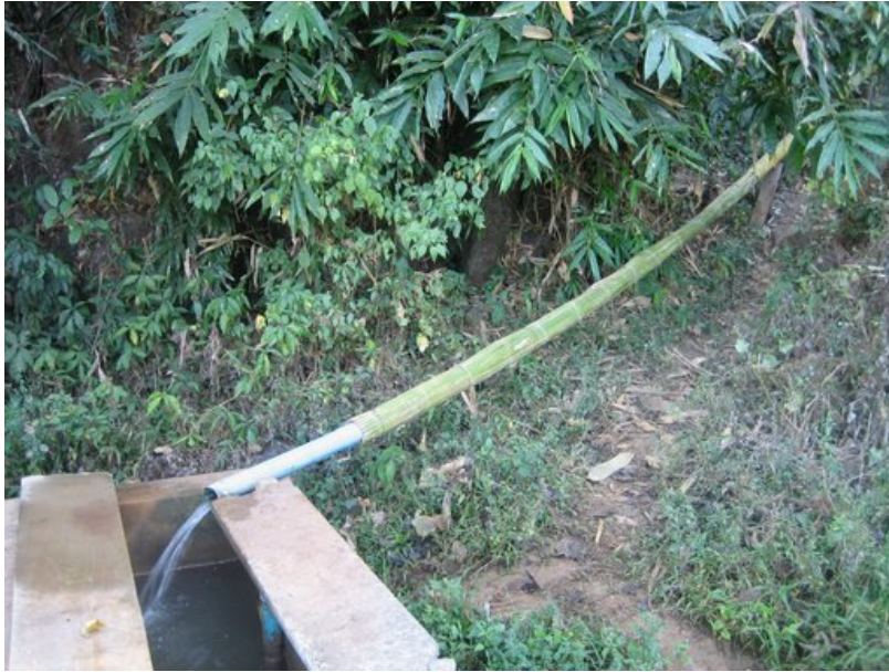
Figure 3-8: Inflow pipe to SP-10 HFRF.
