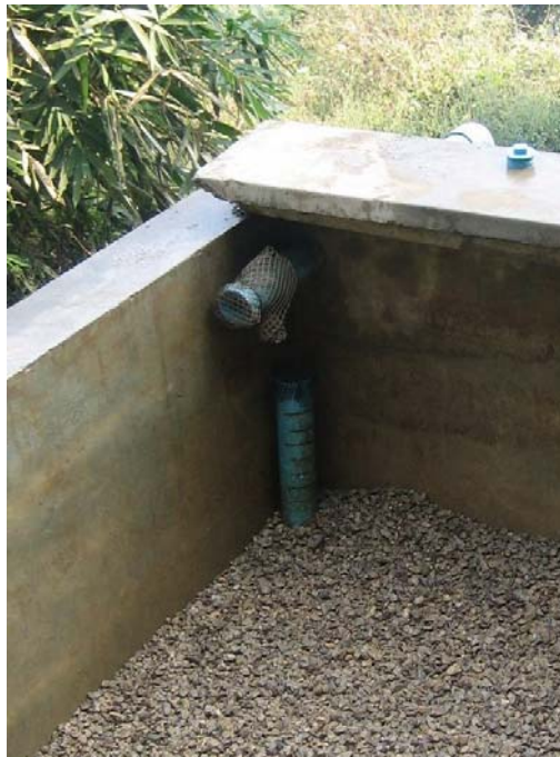
Figure 7-1: Slotted outlet pipe..
