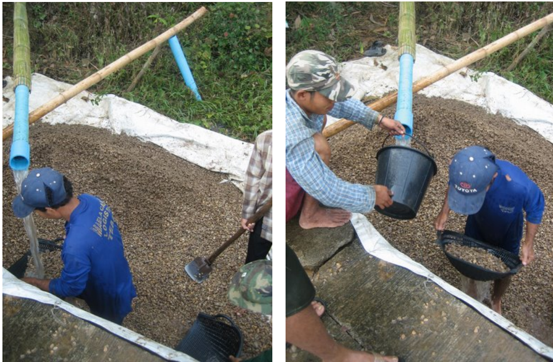
Figure 6-1: Cleaning the HFRF media. (L) Shows the gravel removed from the filter, (R) show the workers cleaning a basketful of gravel with the diverted water supply.
